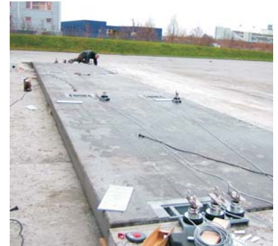
Cablings are drawn to the load cells.
